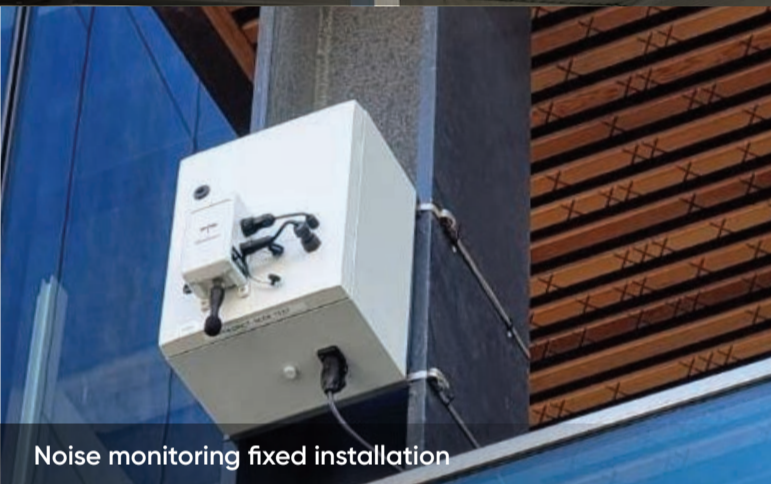
Noise & dust monitoring fixed installation
